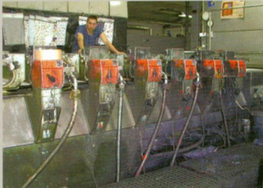
Stork Rd4 before retrofit
